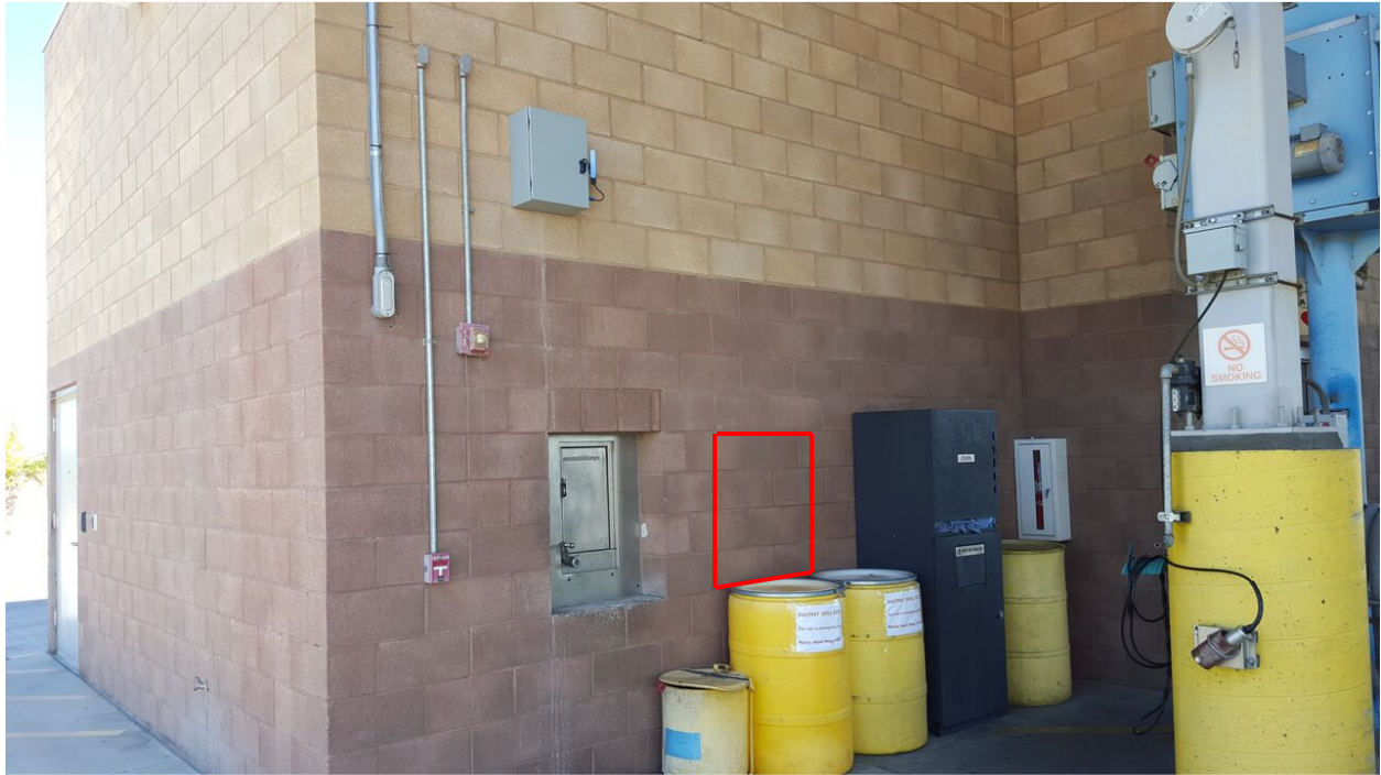
Photo 2 - South Elevation of Coin Operations Building. Proposed new opening shown in red
