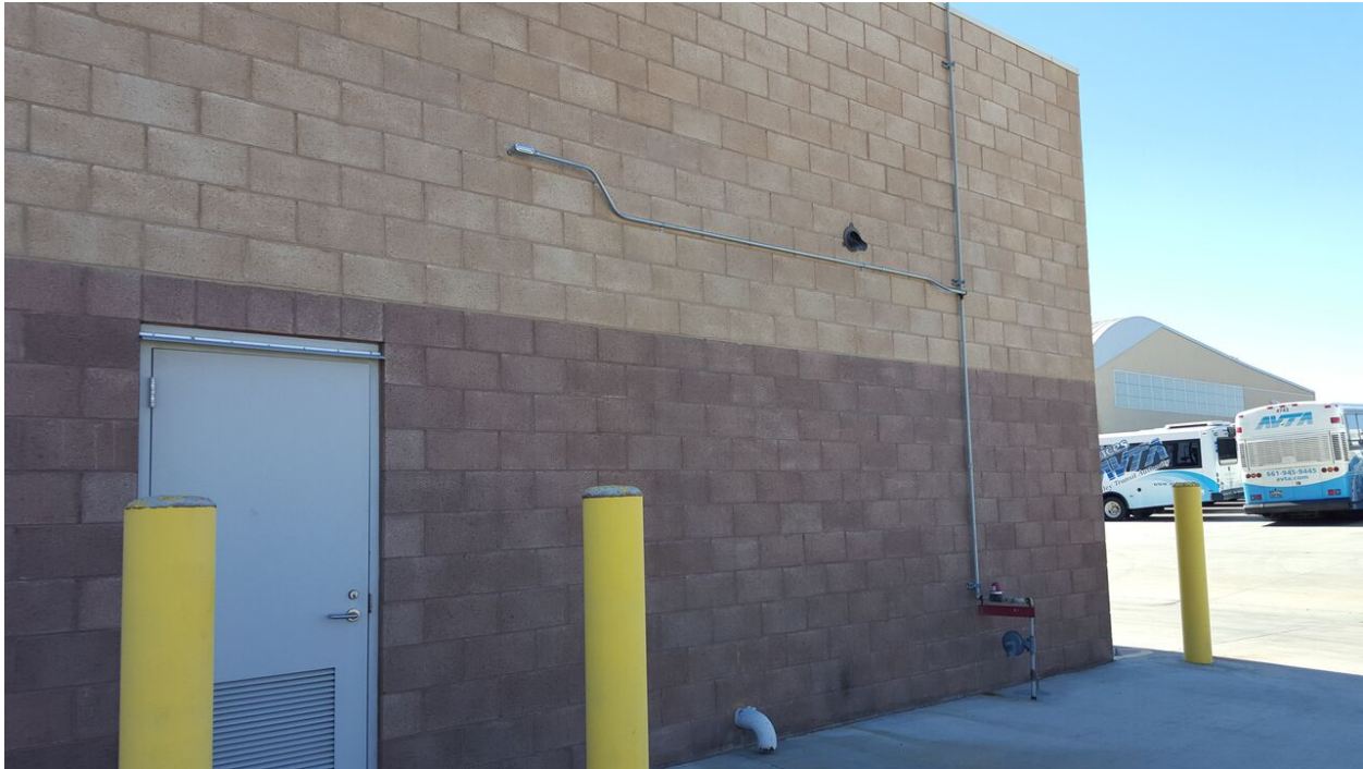
Photo 3 – North Elevation of Coin Operations Building Door shown is existing Electrical Room.
